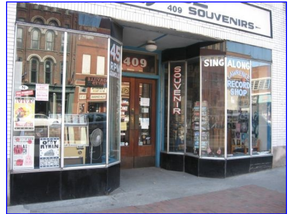
Original display windows like these at 409 Broadway should be retained and, if needed, repaired using materials that preserve their historic appearance.
