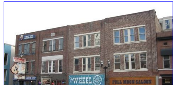
Owners are encouraged to replicate missing cornices where photographic or physical evidence exists. The rebuilding of the historic cornice on this building at 417-423 Broadway as shown below would restore an important design element to the street.
