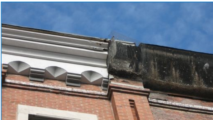
The section of the cornice on the right has deteriorated but originally matched the intact cornice on the left. The missing cornice should be rebuilt to match the existing cornice on the building.
