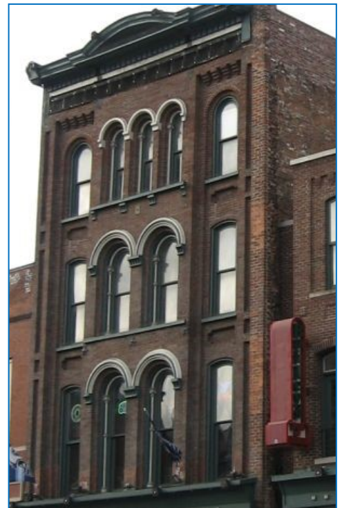
Unpainted stone and brick should remain unpainted unless it was historically painted or if painting becomes needed to preserve the materials.
