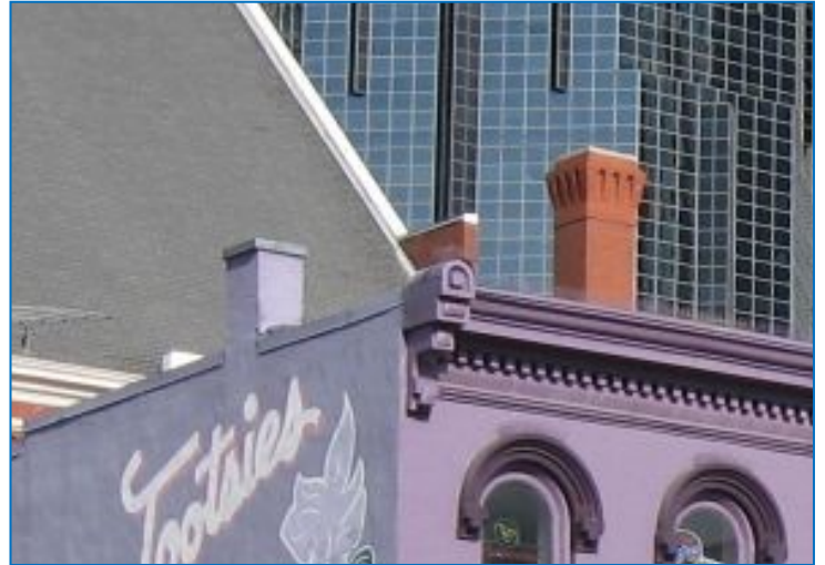
These and other historic chimneys should be retained. They are also appropriate models for replacement chimneys.
