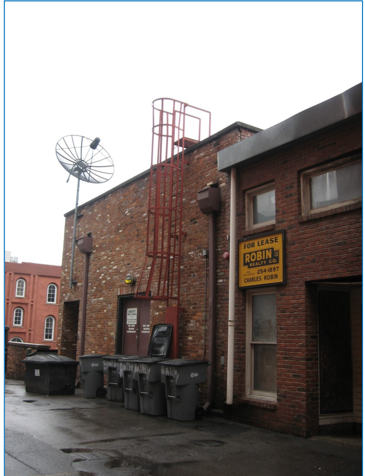
Mechanical units and appurtenances such as satellite dishes should be sited at rear facades.
