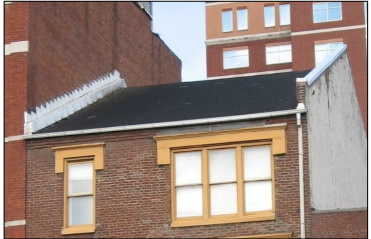
The gabled pitch of this roof is unusual in the district. Its historic pitch and appearance should be retained.
