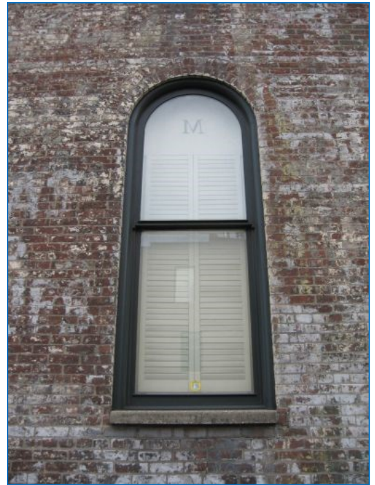
The single-light arched clear-glass panes used in this modern replacement window are appropriate.
