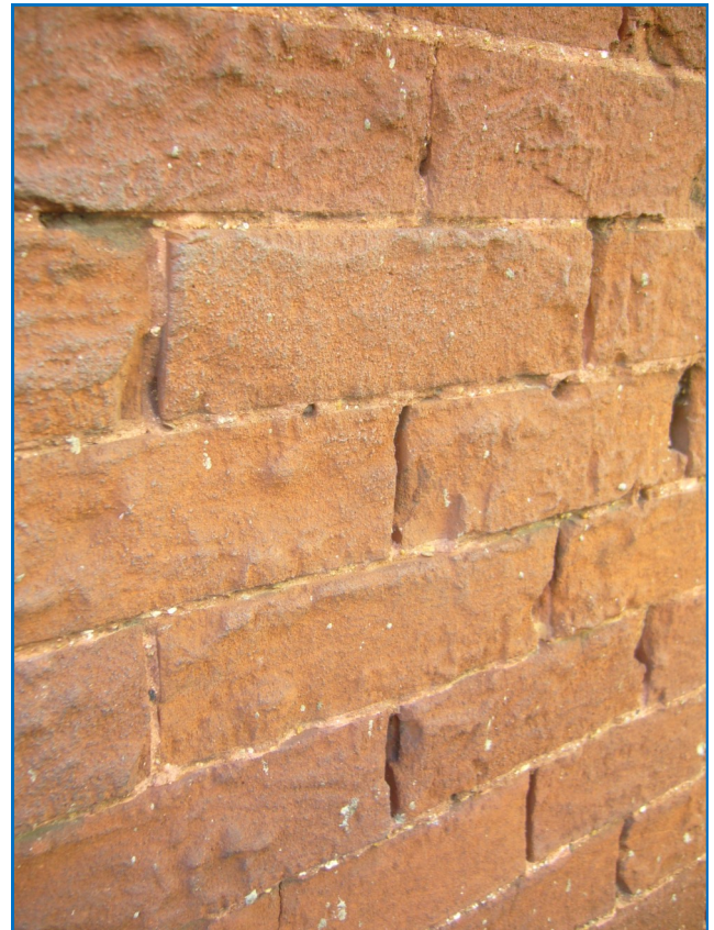
The brick above was cleaned using a harsh method that has removed the hard protective outer surface of the brick.
