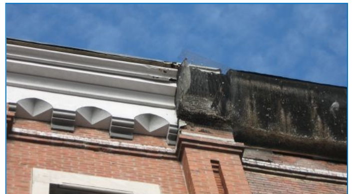
The section of the cornice on the right has deteriorated but originally matched the intact cornice on the left. The missing cornice should be rebuilt to match the existing cornice on the building.
