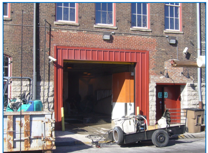
New doors that change the original opening dimensions and design, as seen above on First Avenue, are not appropriate.
