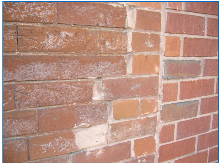
Above is an example of an improper repair that uses bricks of a different color and dimension from the original and the mortar joints also do not match the original tooling.
