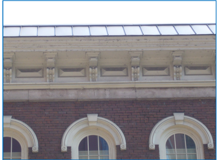
The gabled pitch of this roof is found on some buildings in the district. Its historic pitch and appearance should be retained.
