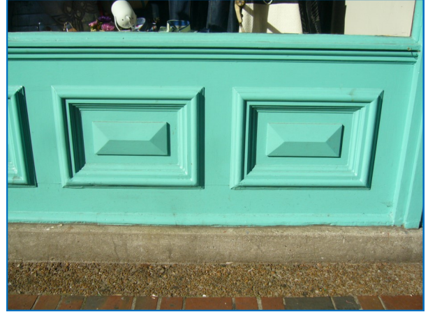
Historic bulkheads should be repaired rather than replaced.
