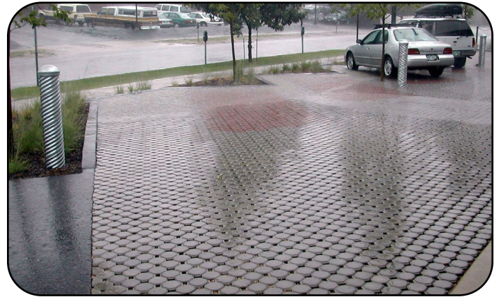
Permeable pavement in parking lot
