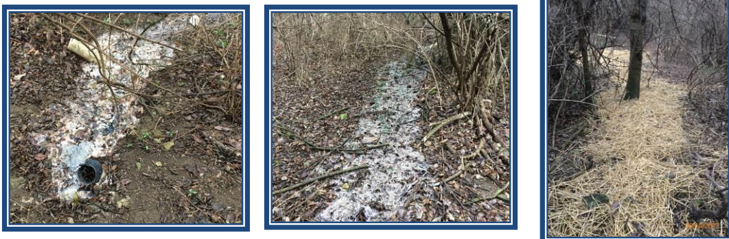
Photographs of the Private Sanitary Sewer Failure
