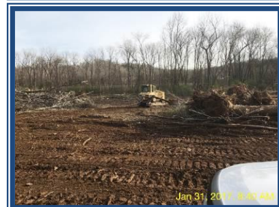
Grading Permit Violation Pictures and Resulting Enforcement
