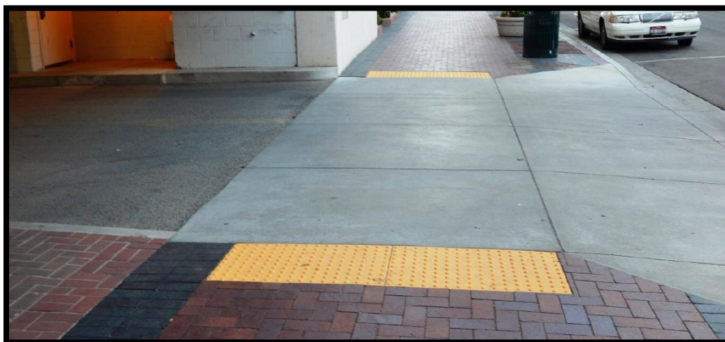
Figure 4-7: Garage Access Ramp Flush with Sidewalk
