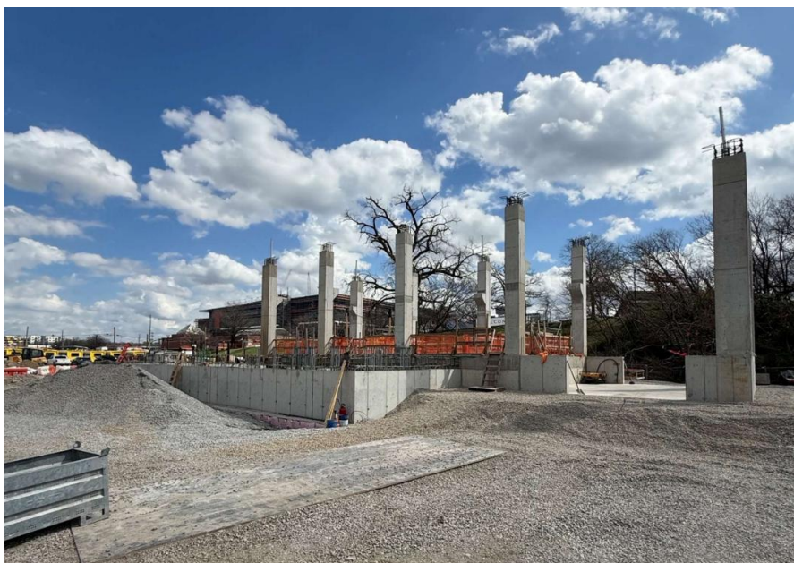
FIGURE 11: LOWER PUMP STATION SITE PHOTO
